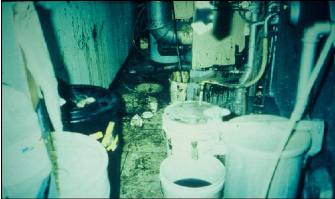
Figure 18. Still Bottoms Discharges. Note the still bottoms spilled onto the floor and splattered on wall behind drycleaning machines.
